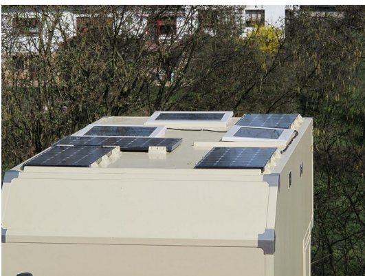
Solar cells and roof hoods
